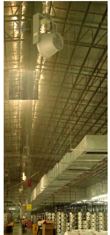
SonicAire® fans keeping plant ducts & ceiling clean
